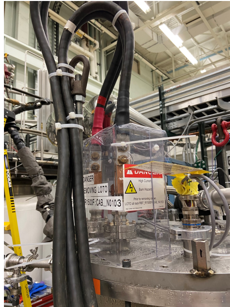
Figure 5.22 500 A power supply DC cable connection to the leads connection lugs of the coil testing assembly.
