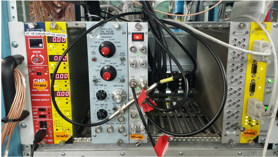
Figure 3.17: All electronics modules utilized on the rack in the S2 vault during NSCL experiment e17024.
